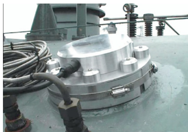
Fig. 2. Externally mounted UHF sensor on the tank of a 1000-MVA, 400/275 kV transformer.
